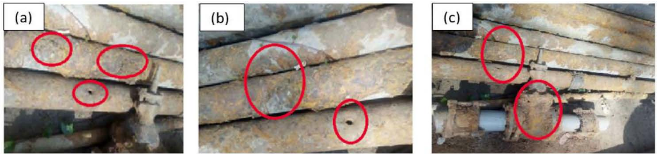
Figure 7: Photograph of corrosion damaged buried water pipes.
